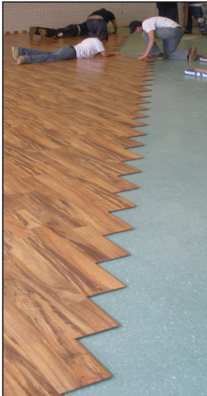
Entrepreneur Program Trainees install a floor on a tribal building, as a practical exercise to learn estimation and bidding procedures.
