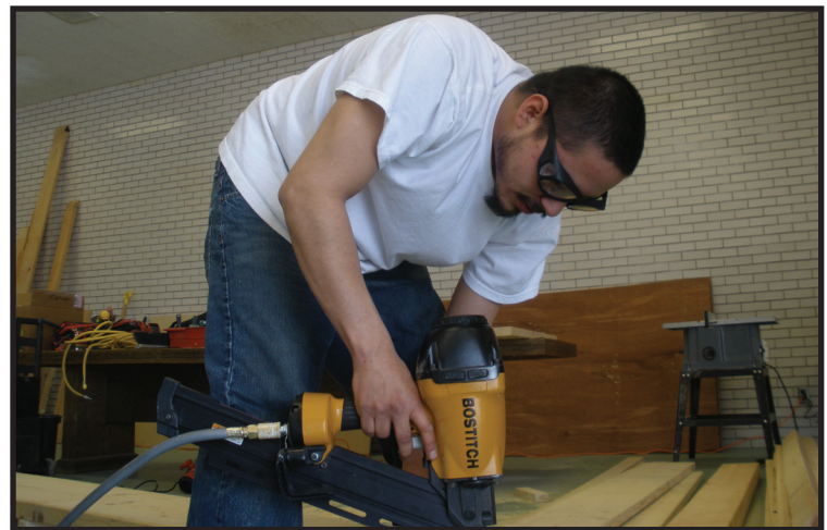
Entrepreneur Class Trainee Kyle Robertson works on a practical project for the tribe during the course of the program. The buildings chosen for NCCI programs are also the classroom sites.
